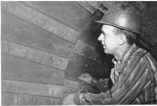
Repairman Ivan Boyce is shown here, inside a ball mill, checking on the installation of new method rubber lining for the ball mill.
