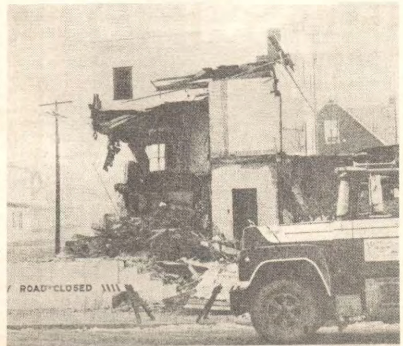
Down with the old-The old city as it is being demolished at the end of October, 1984.
