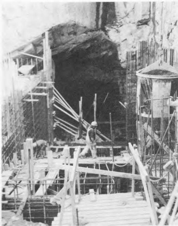
Primary crusher, May 1972
