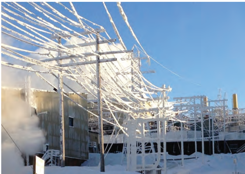
Frosty Power Lines January 10, 2017. Photo by Ken Bateman.
